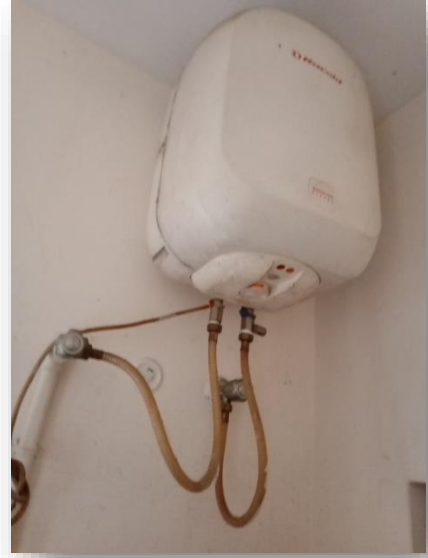
Solar Water Heater
